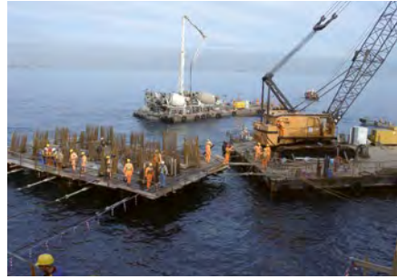
Fig. 8.14.1: When using underwater concrete, the placing and working conditions are very often complex, which is why these concretes often also need an extended working time.
