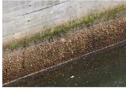
Fig. 8.8.1: Heavy leaching and damage to the structural concrete are observed particularly in the water splash zone of biological treatment basins.
