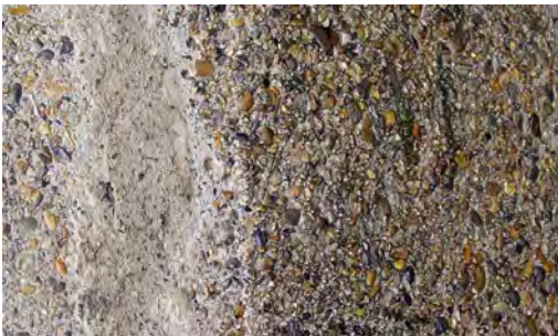
Fig. 8.7.4: Due to continuous exposure, the cement film is eroded in an initial step, and thereafter the aggregates can be rubbed, knocked or washed out of the hardened cement paste.
