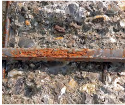
Fig. 8.2.1: Damage to concrete structure due to insufficient concrete cover and low concrete quality
