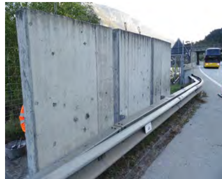
Fig. 8.2.4: Potential measurement on a retaining wall along a road with heavy traffic with high use of de-icing salt, after less than 10 years of exposure. The darker the coloration, the higher the potential for corrosion.
