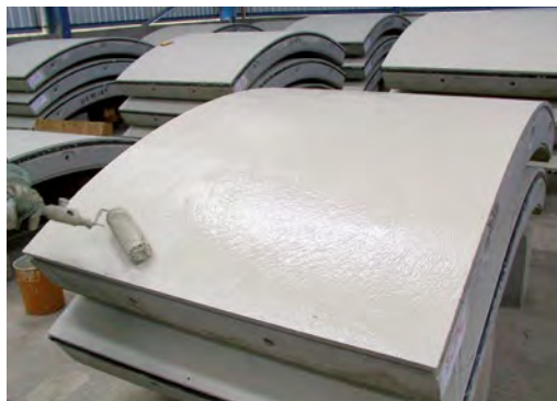
Fig. 8.4.4: Immediately following curing in a steam channel, the concrete surface of tunnel lining segments is coated with water-based epoxy emulsion that is absorbed even into the smallest pores, thereby generating a sealed, protective coating.
